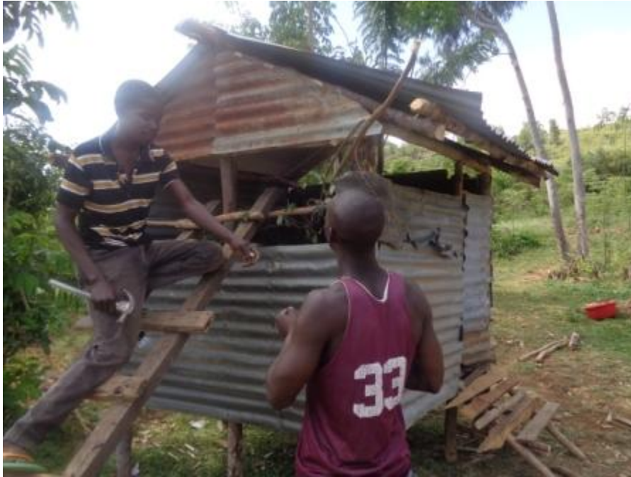
Jared Ouma and Elisha Ochieng relocated Korando D buck unit from Benard Bware's home and reconstructed in Christine Nganya's home
