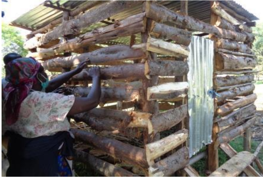
Mary Adede together with other group members – Korando C beneficiary group inspected the newly constructed pure doe unit in Joshua Onoka's
