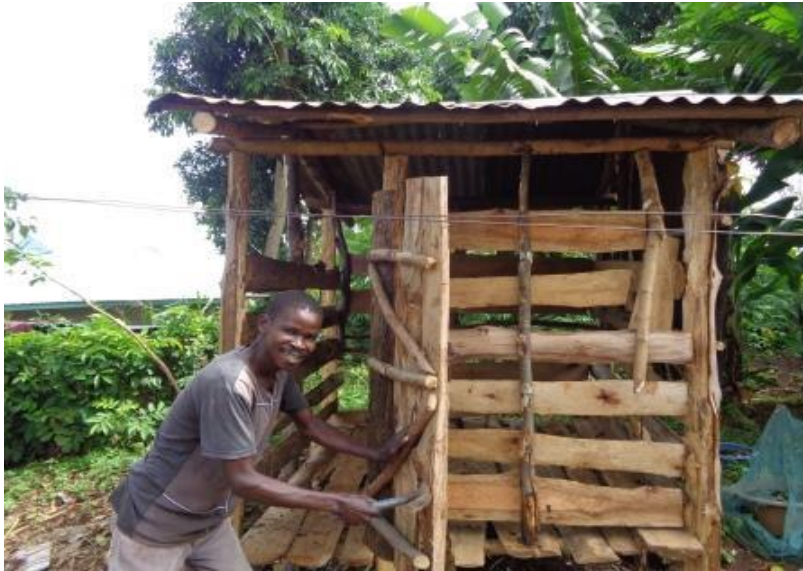
Jared Ouma posed for photo during construction of Korando A buck units in Josephine homestead
